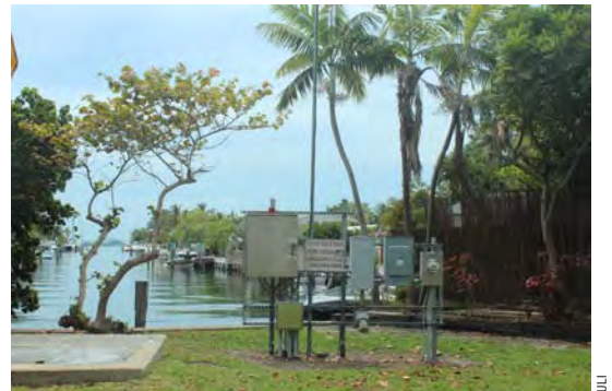
Pumps, pictured here on a waterfront site in the Sans Souci neighborhood, are currently a primary means of dealing with nuisance flooding.
